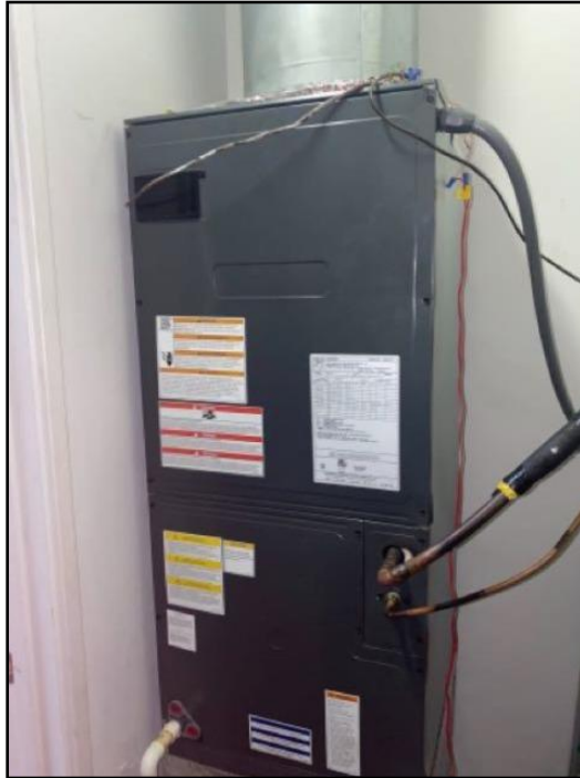
4. Unit#254 Utility Room
