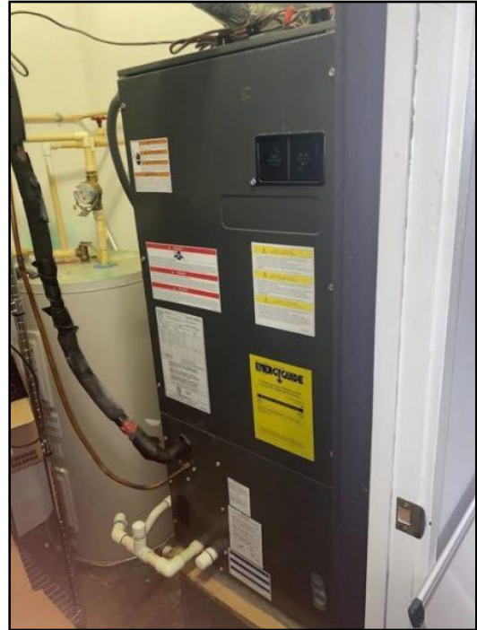
5. Unit#255 Utility Room
