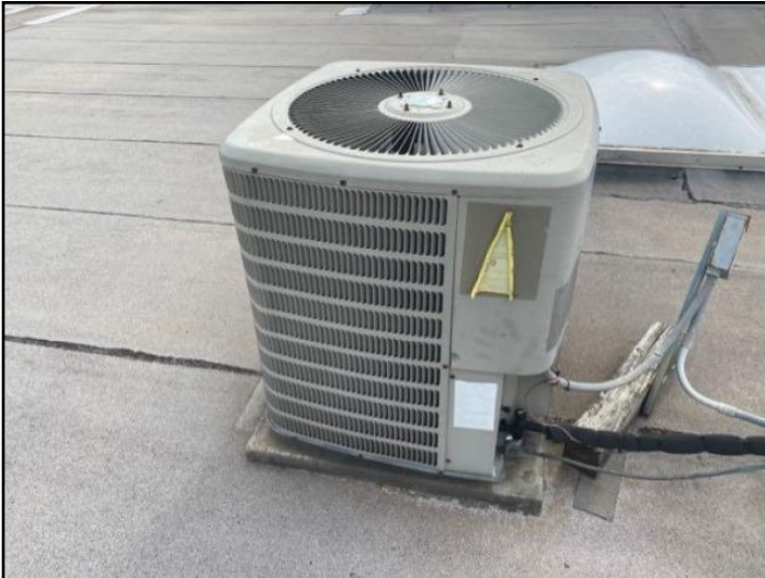
8. Unit#254 Heat Pump
