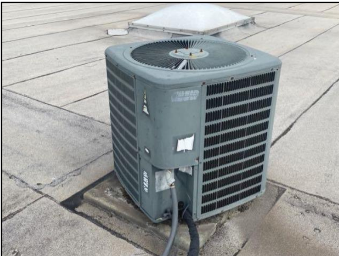
10. Unit#255 Heat Pump
