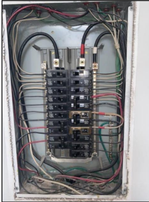
2. Unit 255 - Distribution Panel
