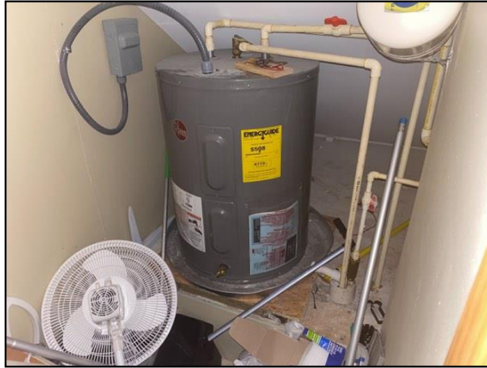
20. Water Heater Unit 2
