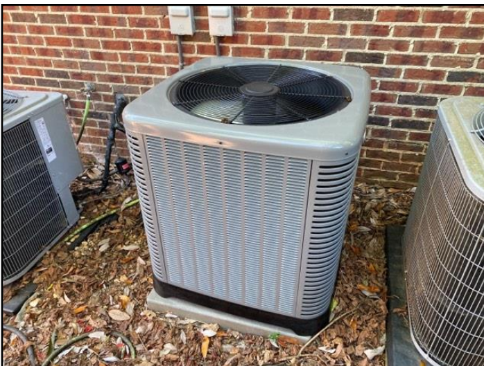
14. Heat Pump Unit 2
