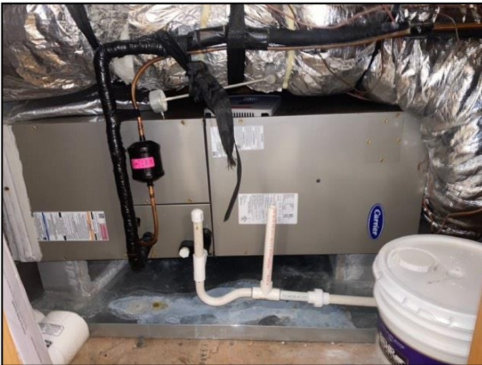
10. Heat Pump Unit 3
