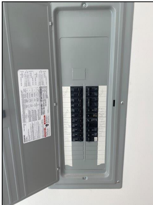
3. Circuit Breaker Unit 2
