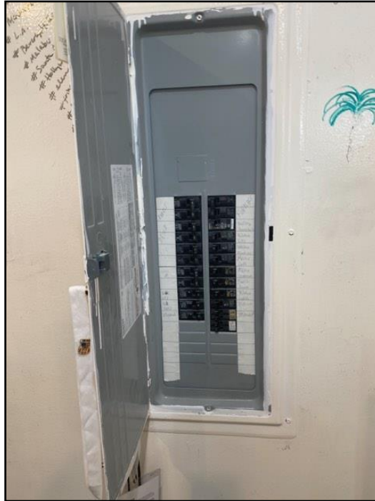
4. Circuit Breaker Unit 3
