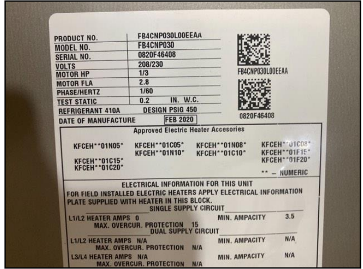
9. Heat Pump Unit 2
