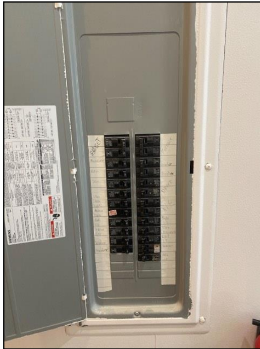
2. Circuit Breaker Unit 1
