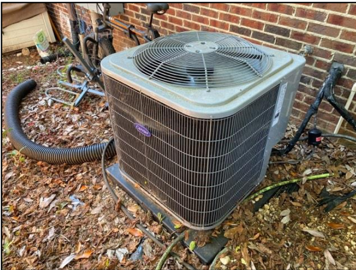
16. Heat Pump Unit 3
