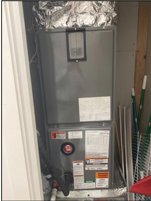
6. Heat Pump Unit 1
