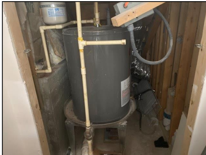
19. Water Heater Unit 3
