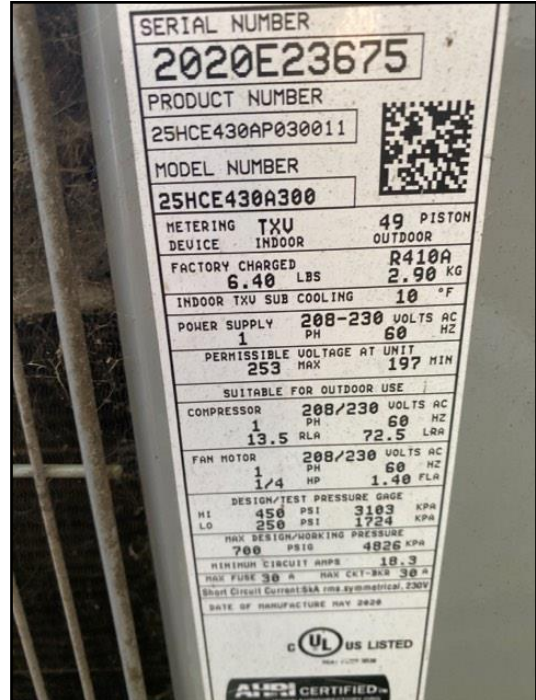
13. Heat Pump Unit 1
