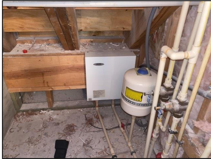
18. Water Heater Unit 1
