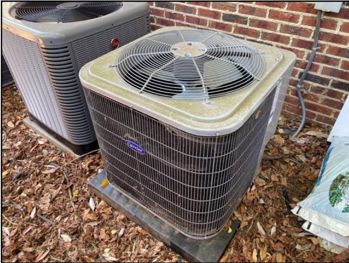
12. Heat Pump Unit 1
