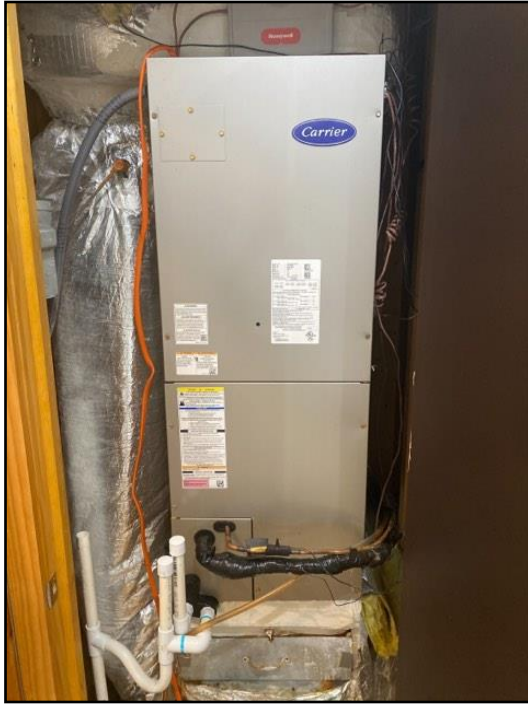
8. Heat Pump Unit 2
