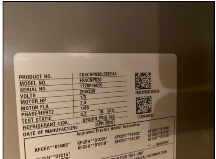
11. Heat Pump Unit 3
